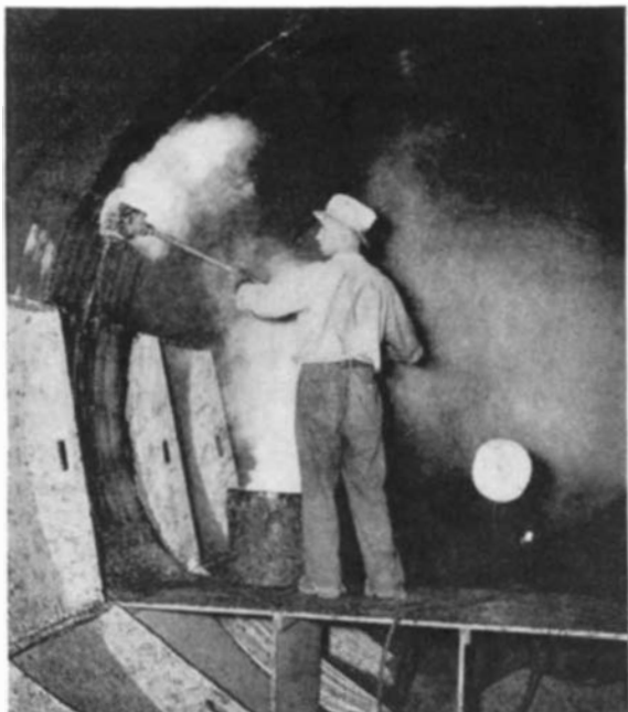
Welded and riveted joints in the steel pipe are further sealed against leakage by an application of hot tar
