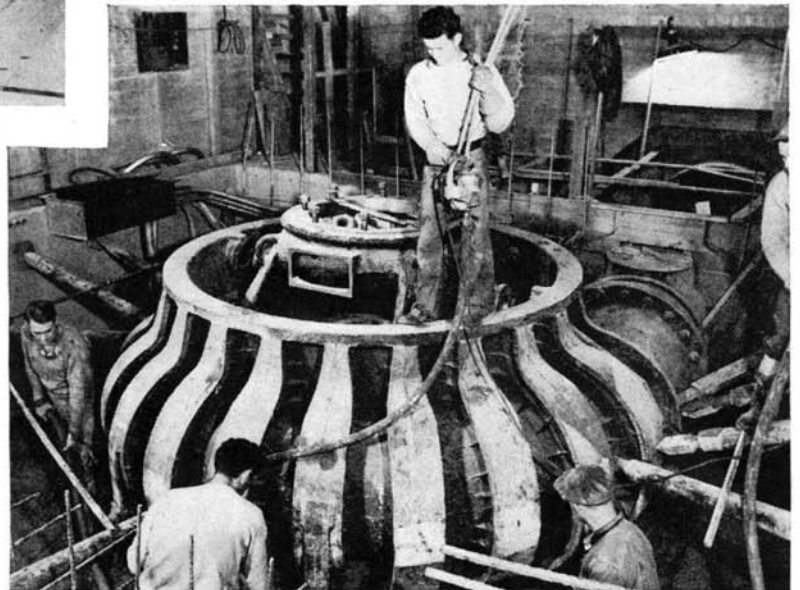
One of the scroll cases within which the impeller of one of the huge pumps will rotate. These cases, placed below water level, will be set in concrete. The impellers will throw water outward and force it upward through pipes
