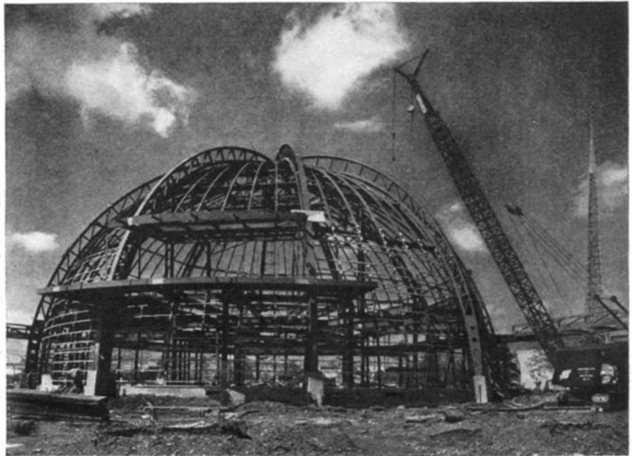
Steel trusses, usually hidden from sight in ordinary building construction, will remain exposed in the "inside out" exhibit building of U. S. Steel at the New York World's Fair. Here is shown the skeleton taking shape, ready to support a stainless-steel dome 66 feet high and 132 feet in diameter. The shape of the building carries out the motif of the Fair's Theme Center which is described in some detail on page 24 and illustrated on the front cover of this number
