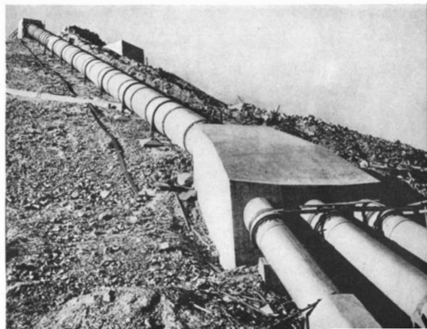
Below: From the intake in the settling basin, water is delivered through three lines to a transition chamber, from which a single pipe leads toward California
