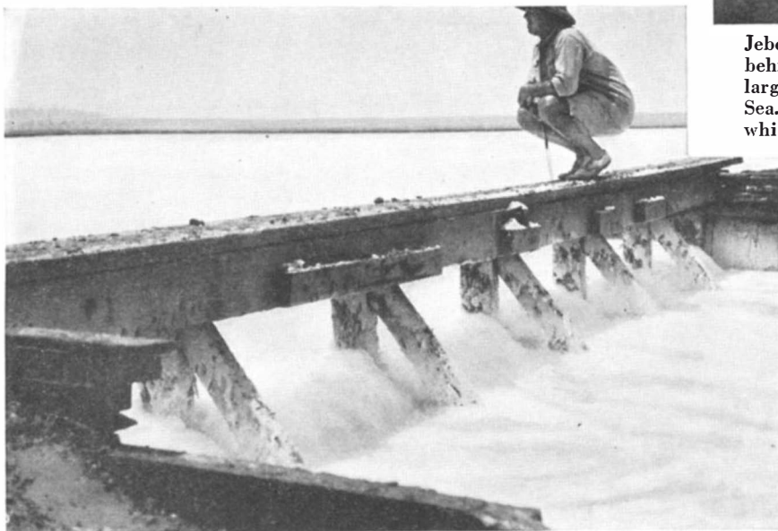
A sluice gate between the pans, by means of which the level of the flow of the brine is regulated. Note the incrustations of mineral salts on the timber work
