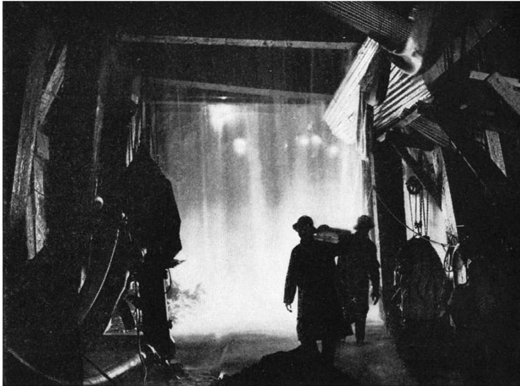
A common sight during the boring of the San Jacinto tunnel was a downpour of water such as this. At one time the inflow to the tunnel at the working face was 15,800 gallons per minute
