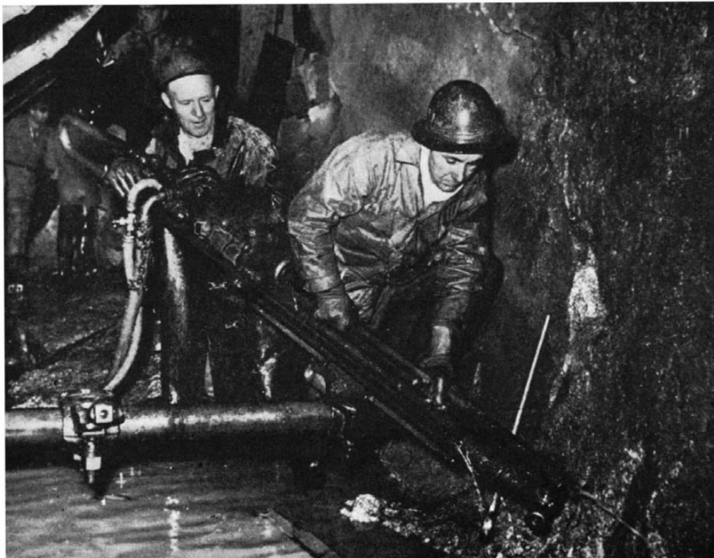
Protected against falling rock fragments by "hard-boiled" hats, and against water by raincoats and boots, the drill workers pushed ahead in the hard rock through which water poured
