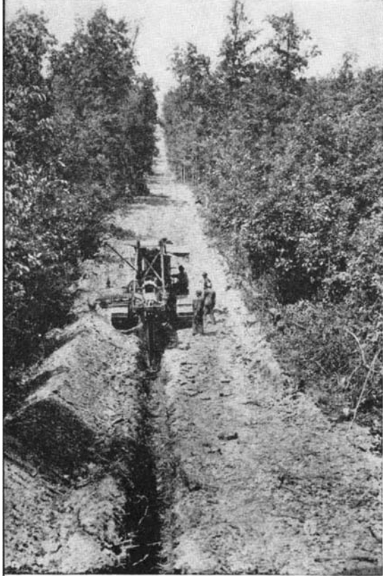
Ditching machine anchored to a tractor and cutting a trench for an oil pipe line on a steep slope
