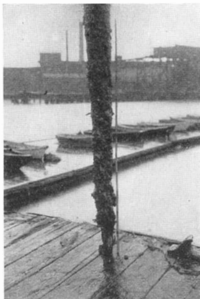
A pile from Chelsea, Massachusetts, showing the result of a heavy marine-borer attack, especially at mud line
