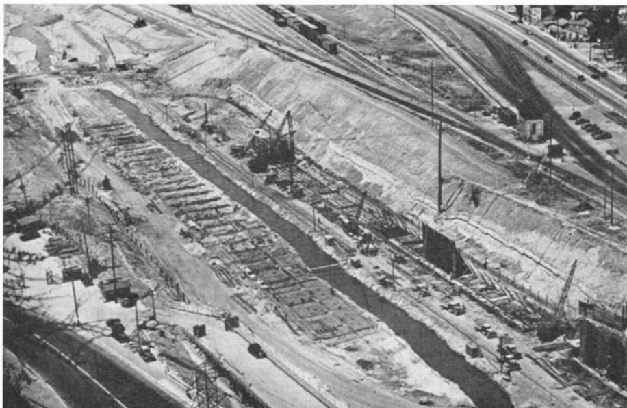
Below: Construction in a congested area, with mountain on one side and railroad yards on the other. The channel bottom is being paved here
