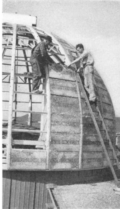
Atop the physics building at the University of Minnesota this 12-ton dome for a 10½-inch telescope is insulated against temperature changes by two-inch slabs of Celotex laid between T-section members
