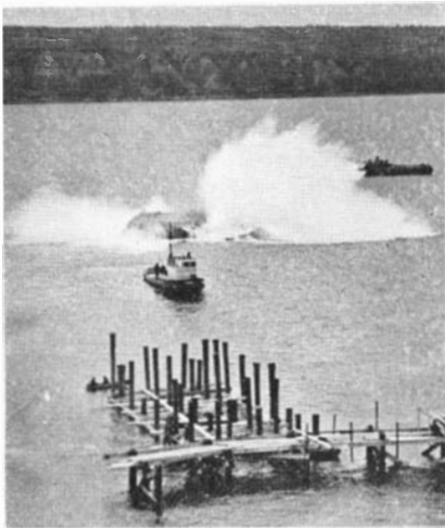
An "anchor" makes a big splash when dumped overboard from a construction barge at a pier site
