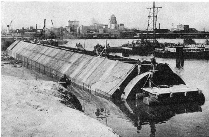
The top of the outer shell of this tube at Blakeley Island is open so that workmen may install wiring conduits, pour the concrete, and so forth
