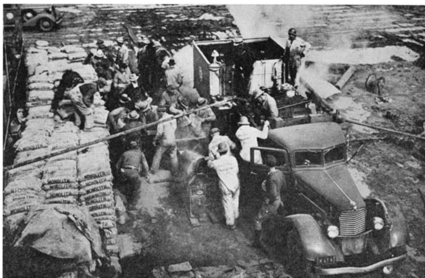
When concreting a deep oil well, men must work at top speed. The mix must reach bottom and return outside the casing before it begins to set
