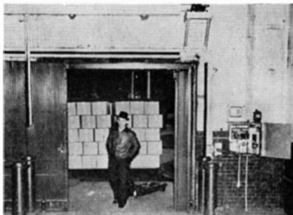
Door-control equipment which saves heating and operating costs in a processing factory
