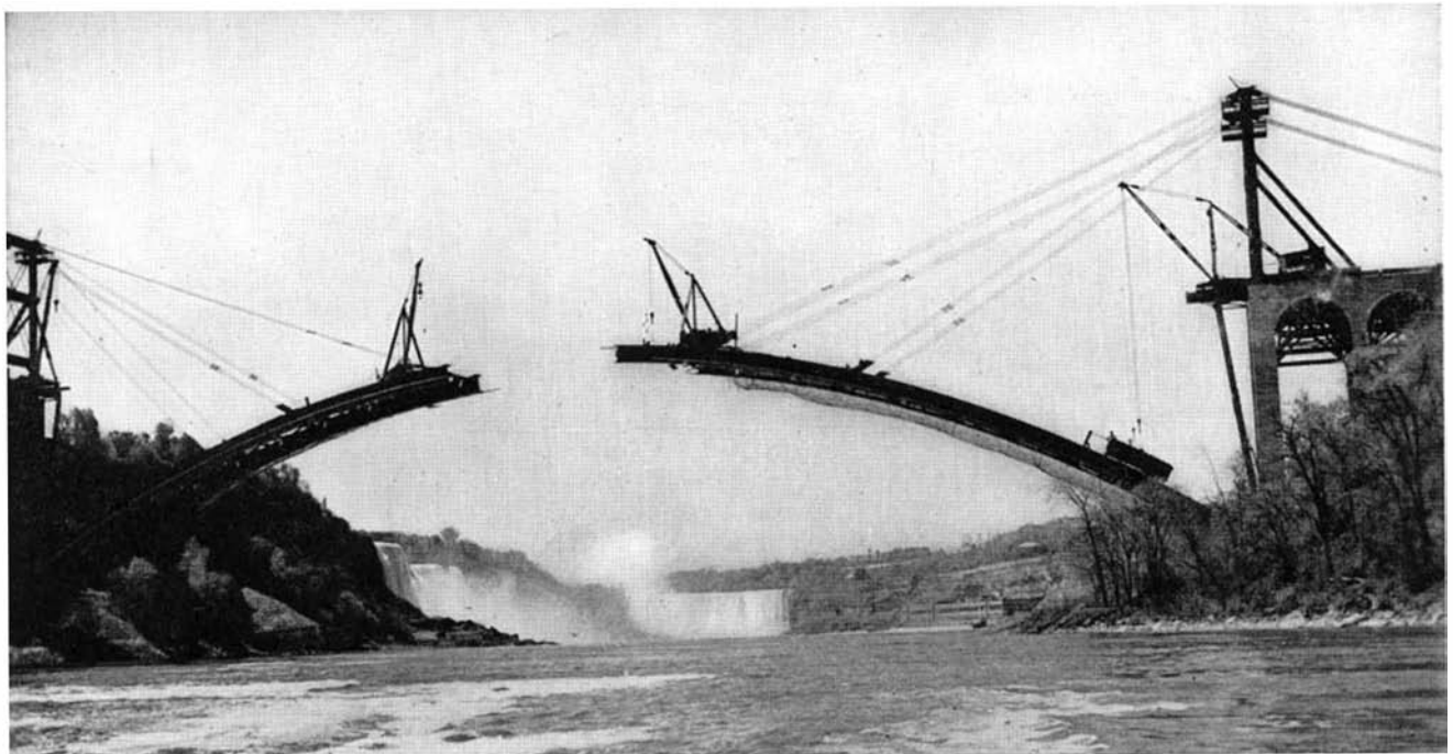
Forming a new frame for an old vista of Niagara's cataract, the 85-ton derricks, on the shore abutments, and the 40-ton derricks, perched high on each span above Niagara River, speed construction of the Rainbow Bridge
