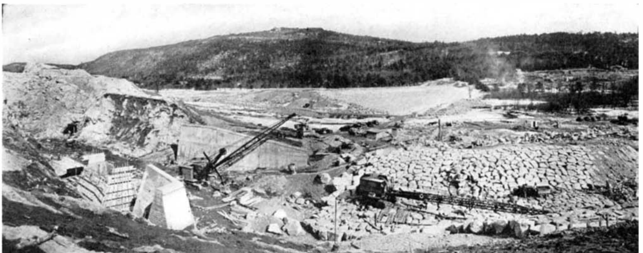
Construction work on Surry Mountain Dam on the Ashuelot River above Keene, New Hampshire
