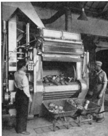
Cleanliness test via open door
