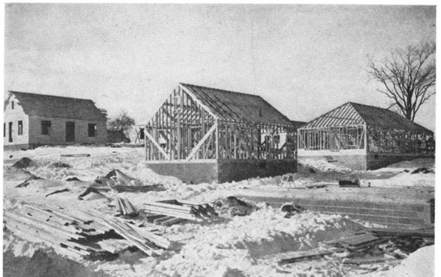
Rough framing of single and double units, and rough boarding of a single unit. In foreground are pre-assembled window frames and studs cut to length
