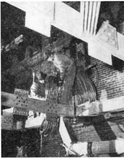
Starter cables to the silver bars
