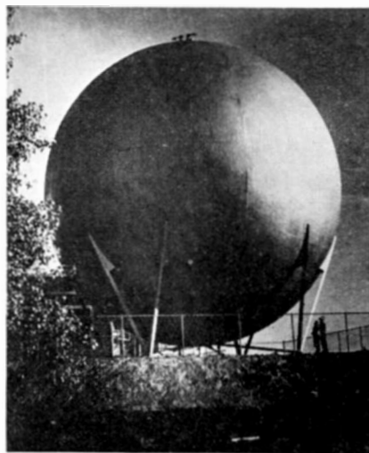
Many modern sewage plants provide storage facilities such as this spherical tank in order to furnish a constant supply of gas for engines
