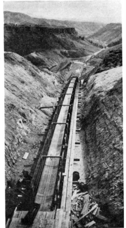
One of the nine long conveyor belts in use at a western dam
