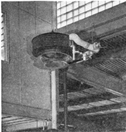
Unit heater which controls winter temperature within 40-foot radius
