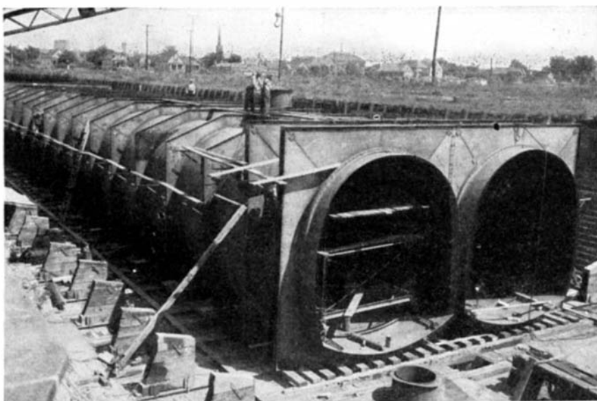
Sections of prefabricated tunnel that now carries the subway under the Chicago River
