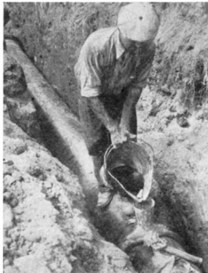
Acid-proof mortar being poured in a joint in a pipe line for disposal of acid waste from an industrial plant
