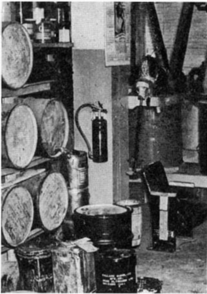
Dry chemical fire extinguishers are spotted strategically in a paint mixing room, ready for instant use
