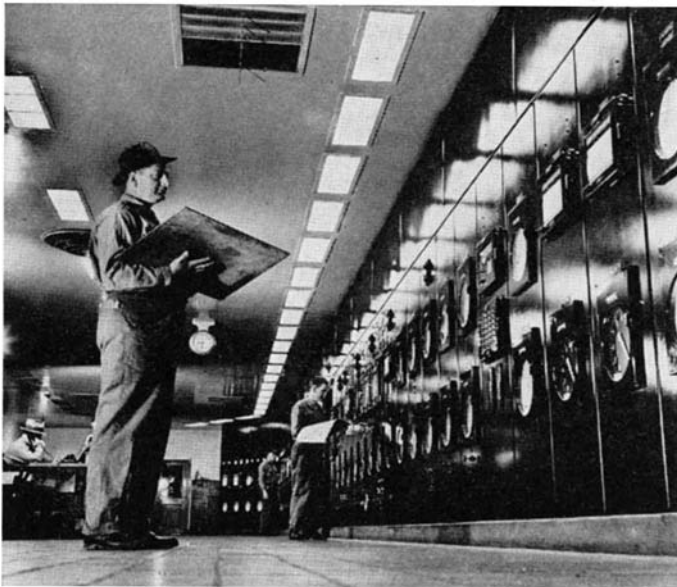
Courtesy Standard Oil Company (New Jersey) Control room of a fluid catalyst cracking plant
