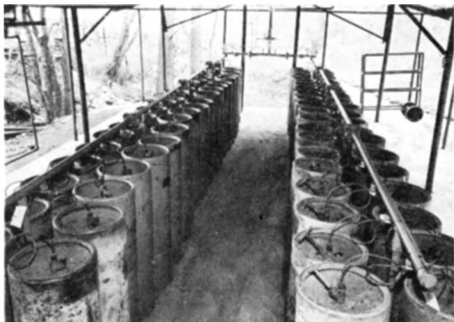
At a war plant, batteries of 100-pound tanks of LP-Gas are manifolded to supply ample gas at required pressure
