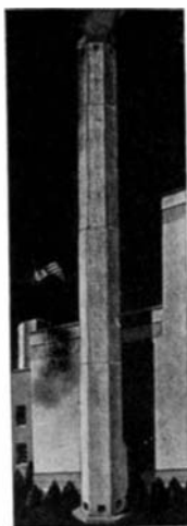
High efficiency insulated smoke stack
