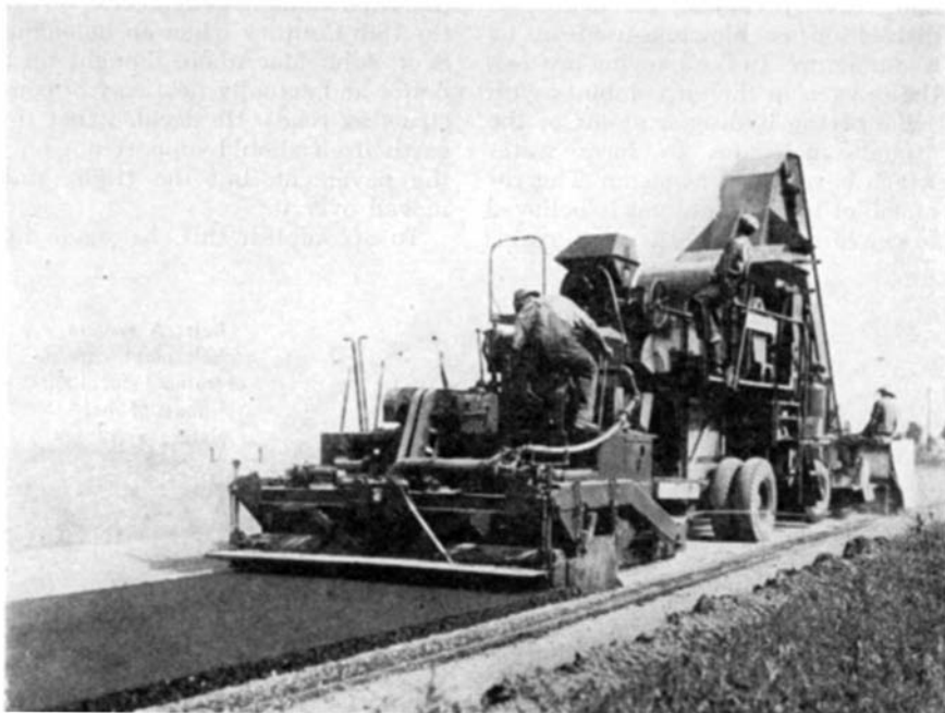
This modern road-building machine scoops up the materials laid out before it, mixes them with asphalt in the desired proportion, and spreads the finished product
