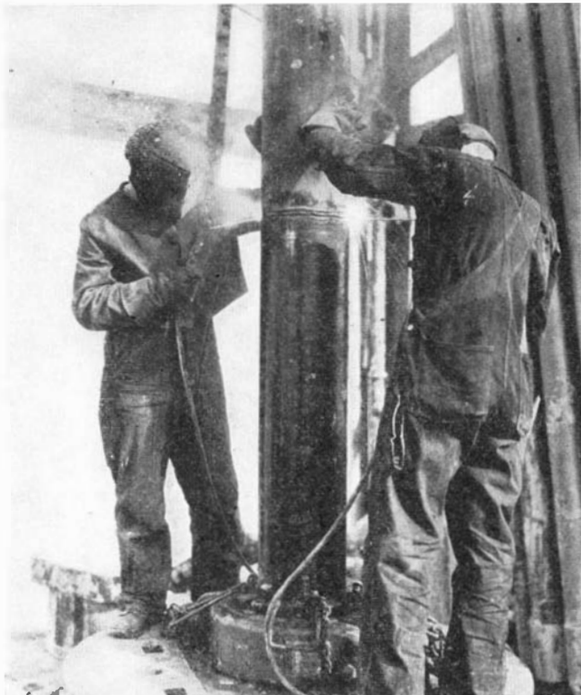
Two men working on one weld must have their operations timed so they can work efficiently without mutual interference
