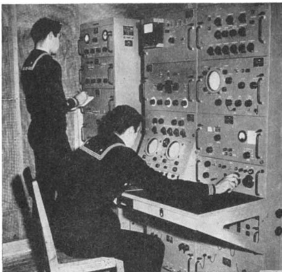
Interior of Loran transmitting station where operators maintain constant watch on timing equipment. About 150 such installations could cover the main travel routes of the world
