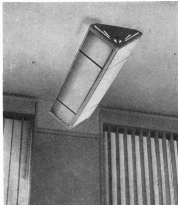
School-room light meter (above) fixed to monitor's desk, tells when extra, or less, light is needed from fluorescent lamps (left). Louvers on windows in the background control sky glare, team with asymmetric light distribution from lamps to boost blackboard visibility
