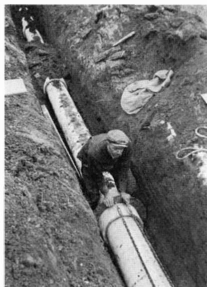
Asbestos-cement pipe in 13-foot lengths is joined together by sleeve couplings made of the same material. Hydraulically operated puller is used to draw the coupling over the ends
