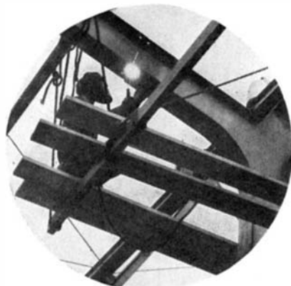
Courtesy Lincoln Electric Company Supervision Required
