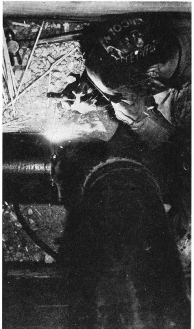
Not a single welded joint in a mile of pipe in a factory steam distribution system showed even a pinhole leak under hydraulic test at 400 pounds gage
