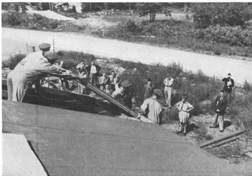
Removing the roof from one of the Canadian Army's demountable, prefabricated "hutments." The demounted hut is light and small enough to be transported by air
