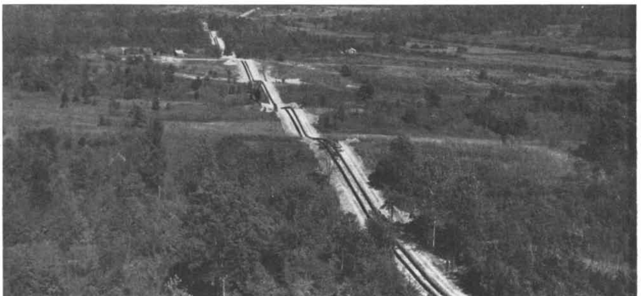
NATURAL GAS PIPELINE of the Texas Gas Transmission Corporation lies beside its trench in the hills of
