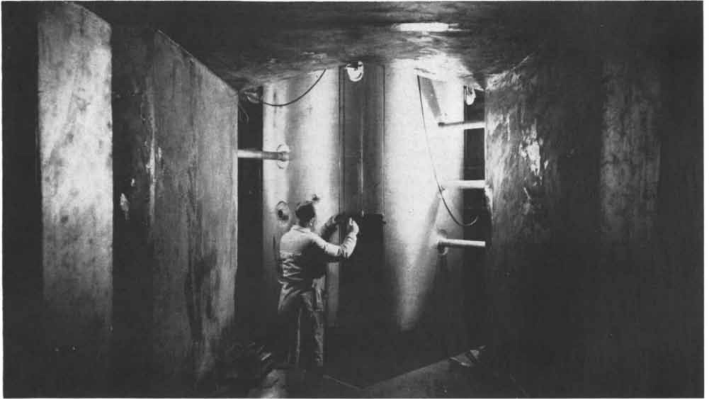
ALUMINUM TANK is seen during the construction of the reactor through an opening in its concrete shielding.
