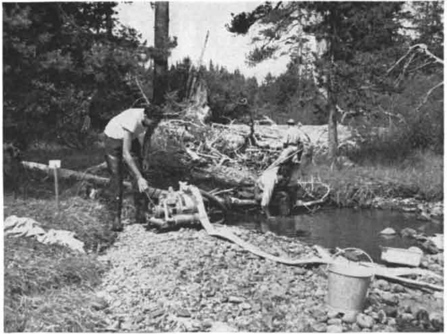
WATER IS PUMPED from a section of Sagehen Creek by building two dams and routing the stream around them. One dam is in the background.
