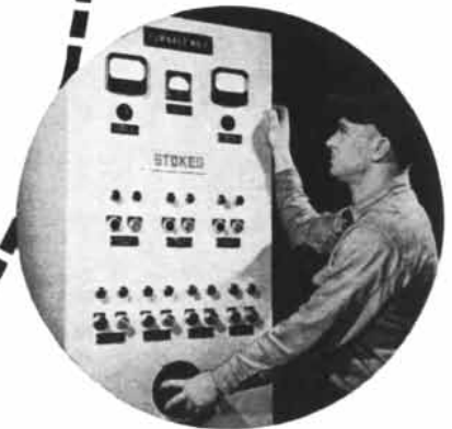
Operator regulates booster pump from central control panel. This is one of a battery of 16 Stokes Vacuum Furnaces in a major installation.
