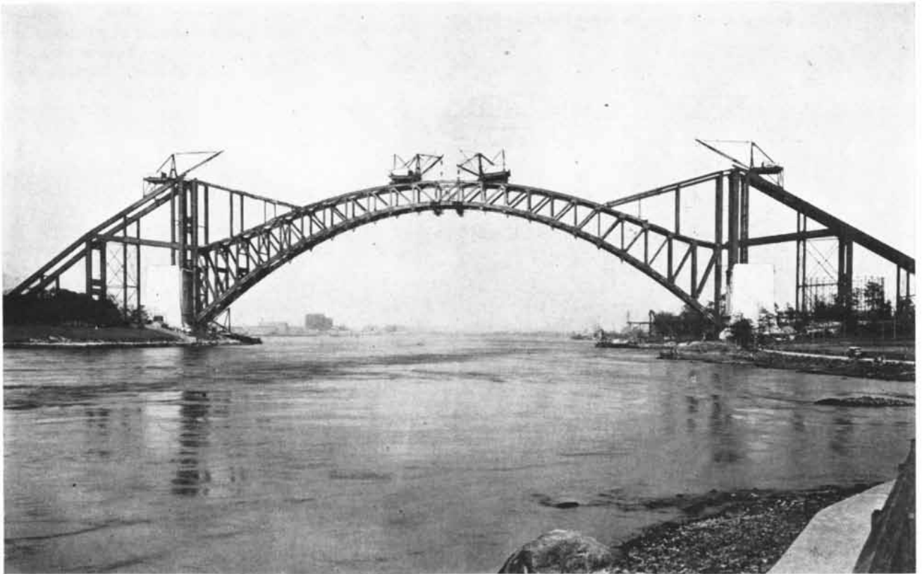
HELL GATE BRIDGE , which crosses the East River in New York, has a span of 977 feet. Here it is shown during construction in 1915. Because the water was too deep and swift to permit the erection of scaffolding, the two halves of the arch were built out from the ends.
