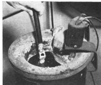
Fig. 1. This photograph shows an aluminum cable being soldered by immersion in a bath of molten solder. Using fluxes developed by Kaiser Aluminum, it is as easily dip soldered as the most soluble metals.
