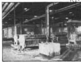
Small section of filtration floor in new plant addition.
