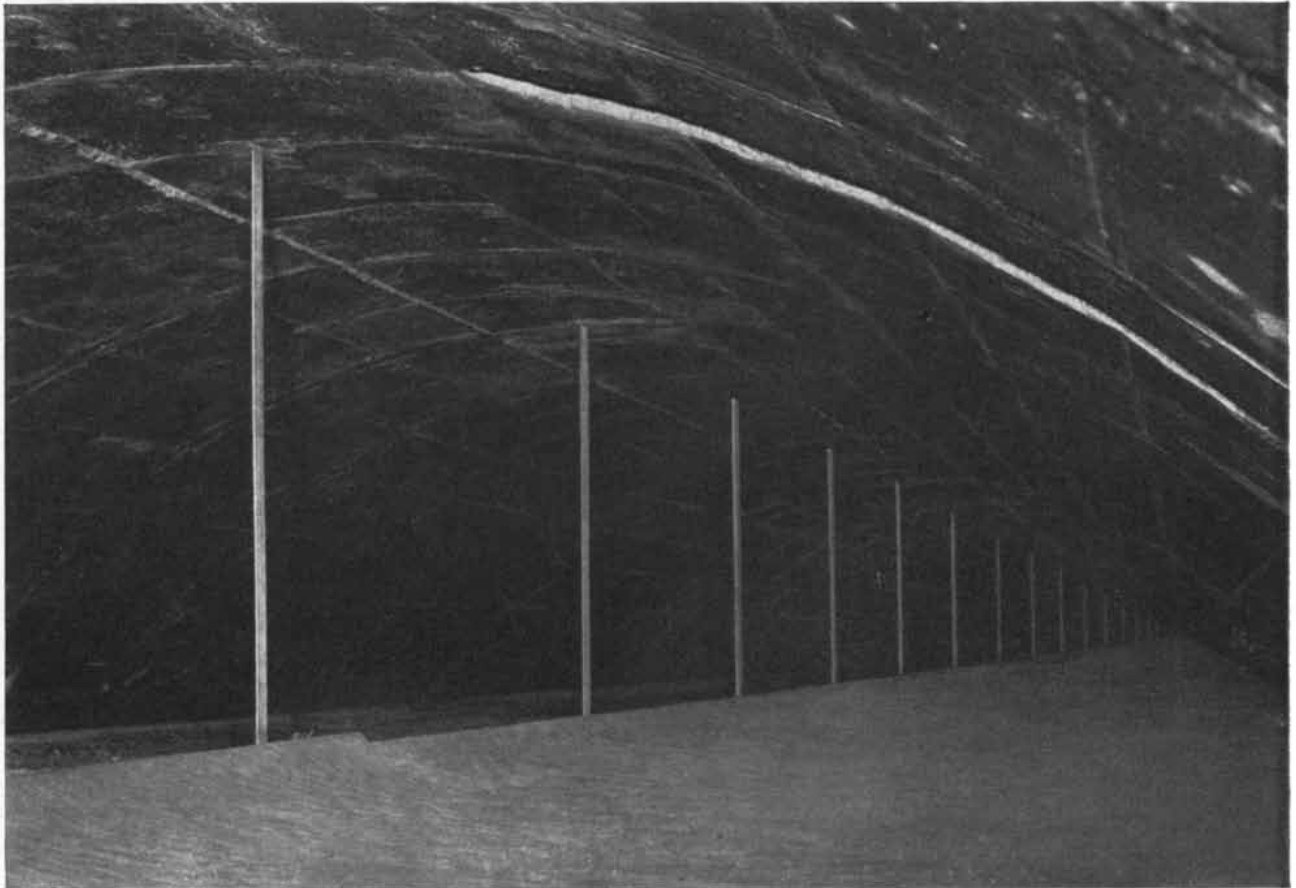
Tunnel within a tunnel — 8500 ft. exhaust ducts are supported by seven-foot Monel hangers. There's one every eight feet along the duct.
