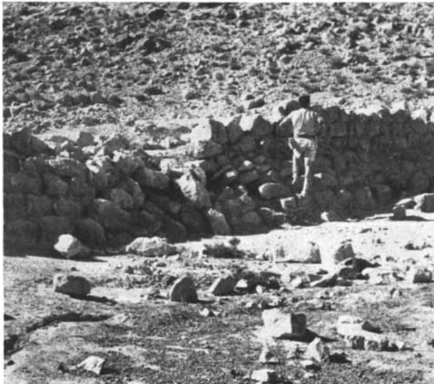
STONE WALLS controlled the flow of water in the wadis. The photograph at the left shows a low dam with a damaged spillway.
