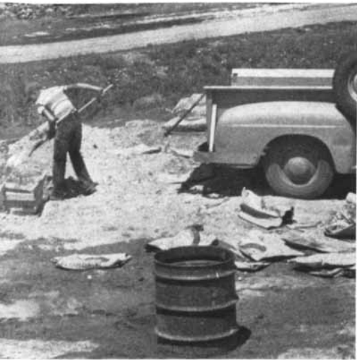
the assets of the Mormon community. Volunteers here mix concrete for foundations.
