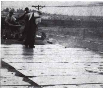
Food Fair Company's new frozen-food warehouse in Linden, N. J., uses vapor barrier made of Du Pont "Mylar" and foil. The barrier is easily applied and sealed tightly with pressure-sensitive tape of the same material. Men shown walking on the vapor barrier illustrate the extra toughness and abrasion resistance of this lamination with "Mylar".
