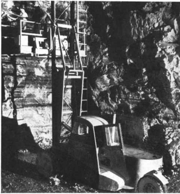
OIL-SHALE MINING methods were developed by Bureau of Mines engineers at Rifle, Colorado. The picture shows mobile platform used for charging blastholes in the working face of the mine.
