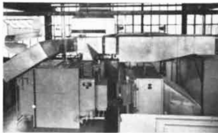
This Lectrodryer works with refrigeration equipment to condition the air in our engineering department.
