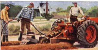
To conquer the wind, Anaconda Direct-burial Telephone Cable was installed on Ocracoke.
