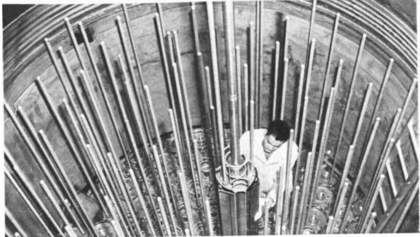
Reactor "heart" . An AI technician installs zirconium "cans" containing the graphite moderator in the core of the Sodium Reactor Experiment. The use
