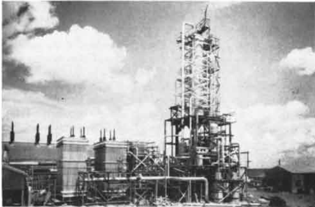
Photograph shows installation of Alcoa Aluminum equipment and piping in oxygen plant detailed in flow diagram. Harp-type heat exchangers (left) are dip-brazed assemblies with thousands of fins for best heat transfer.
