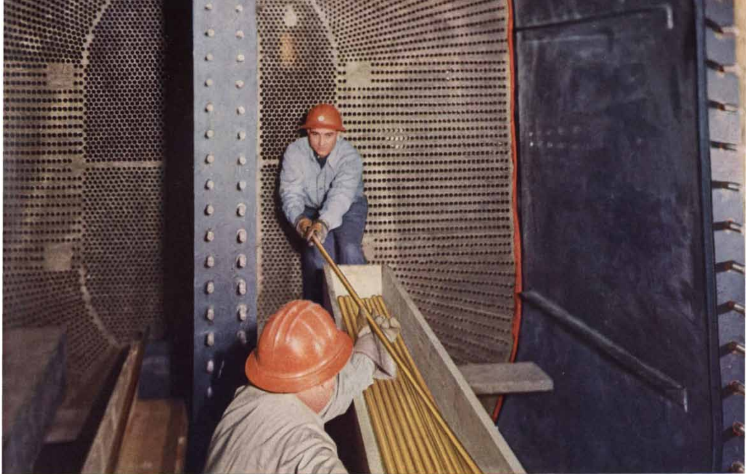
10,276 Anaconda Tubes, 7/8" diameter and 30 feet long, were inserted in 1/2"-thick, 6-ton Anaconda Muntz Metal plates of condenser at Shippingport.
