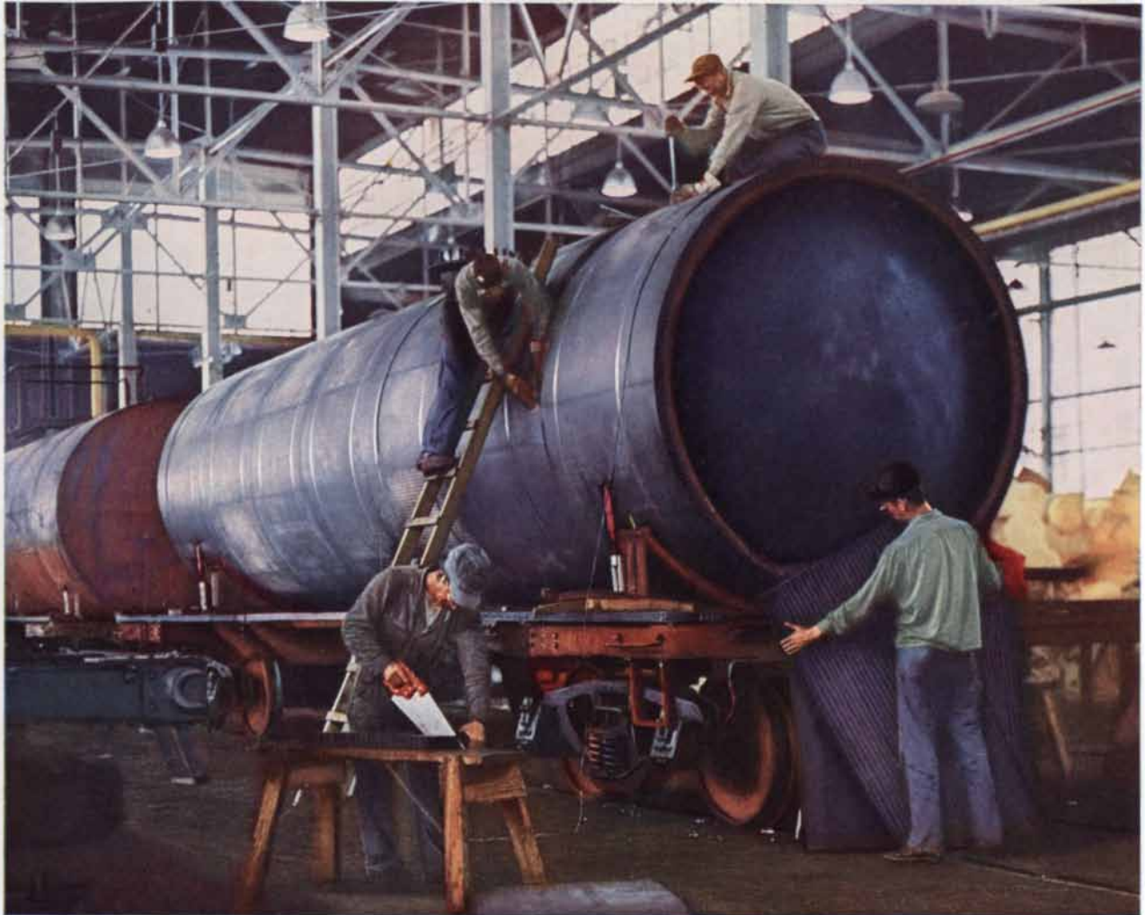
Photo courtesy Union Tank Car Company, Chicago, Illinois. Insulation hardboard supplied by Rubatex Division, Great American Industries, Inc., Bedford, Virginia
