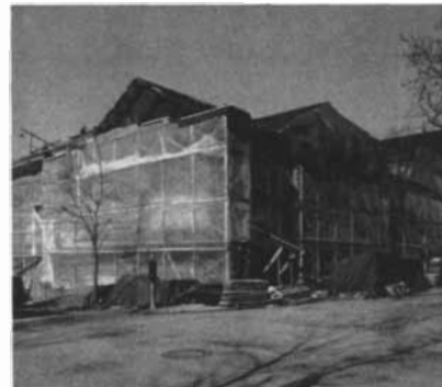
SNUG IN 60-MILE-AN-HOUR GALE, workmen continued building Brown University dorm. Construction was "gift-wrapped" in polyethylene film.
