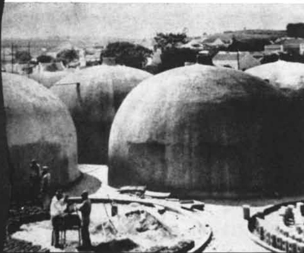
Concrete storage houses built on pneumatic forms, fabricated by Goodyear Tire and Rubber Company, using a Wellington Sears nylon base fabric.
