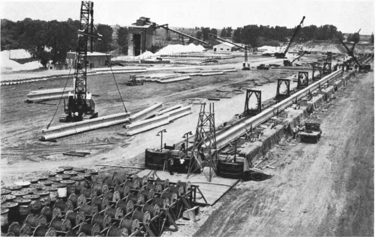
PRE-TENSIONING PLANT of the Material Service Corporation in Chicago makes prestressed concrete beams for bridges. At lower left are reels of cable which feed three production lines 600 feet
