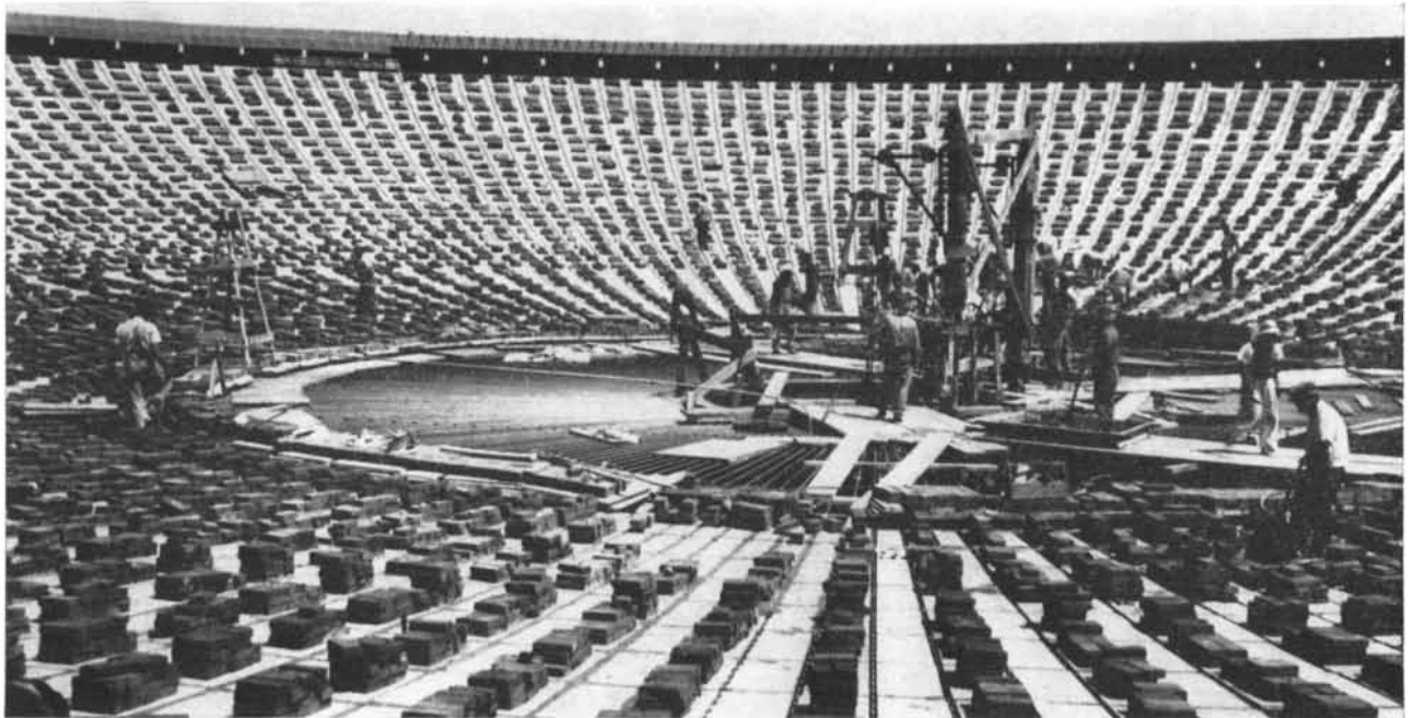
ROOF in Montevideo, Uruguay, was designed by the Preload Company. Small slabs of concrete are suspended from radial cables.
