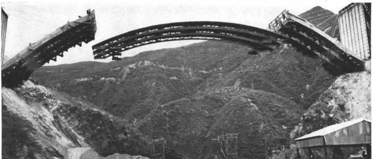
SPAN made of prestressed concrete sections is lifted into position to make the arch of a bridge on a highway which connects Caracas,
