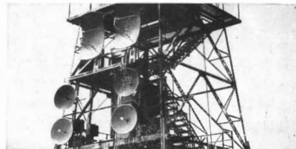
WORDS OR PICTURES are beamed cross country by microwave relays eliminating wires and damage from storms. Western Union system using Sperry microwave tubes handles up to 2,000 messages simultaneously.
