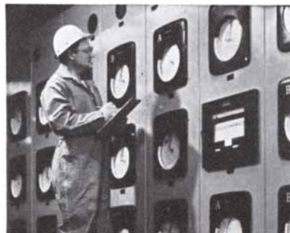
Pinpoint temperature control in 350°F-750°F range can accurately be achieved with Dowtherm.
