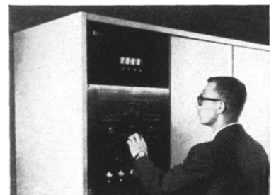
Typical 2000 point system delivered to a major nuclear propulsion test facility.
