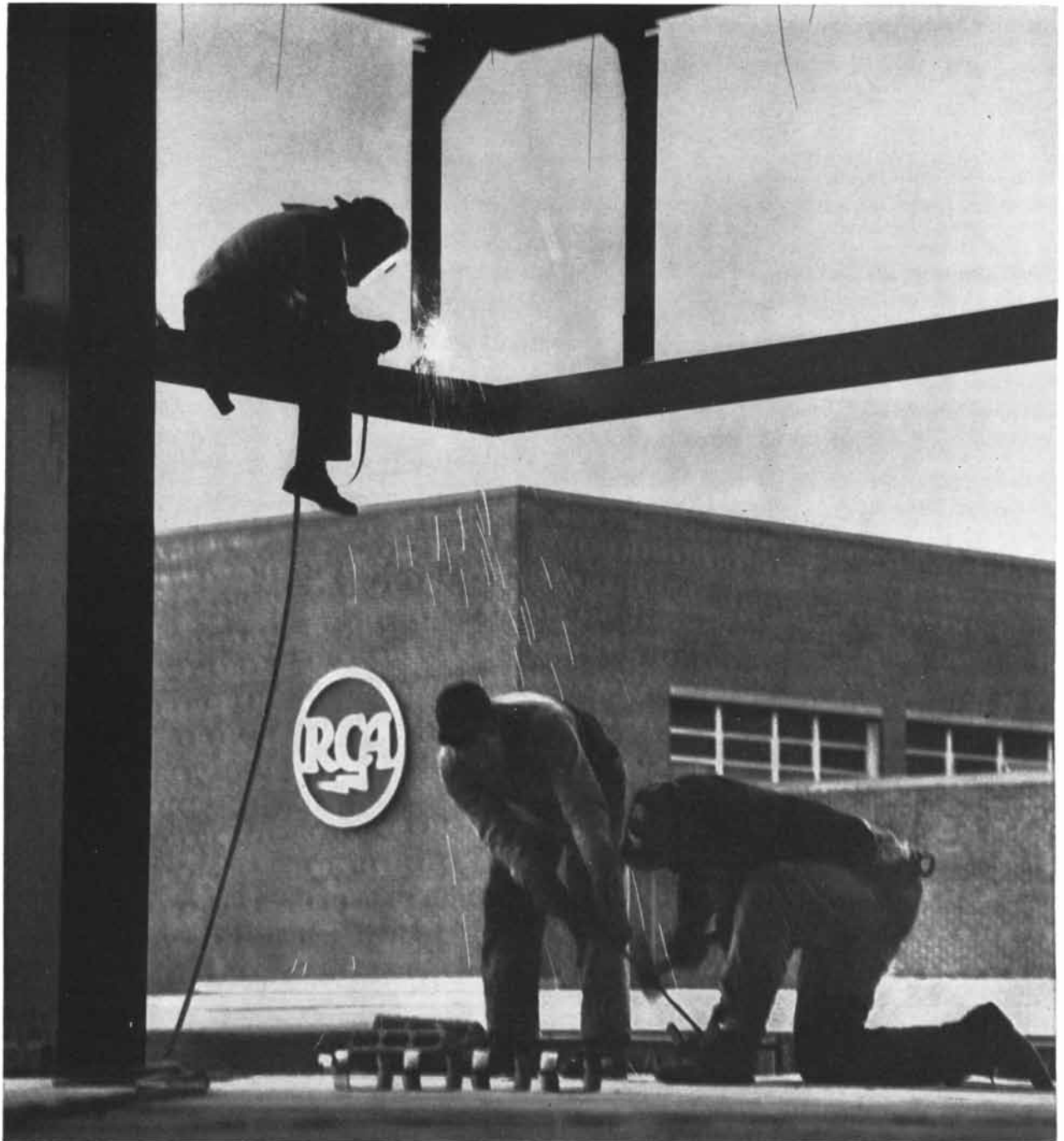
Construction of additional building in progress at RCA Moorestown—to be completed Spring, 1960
