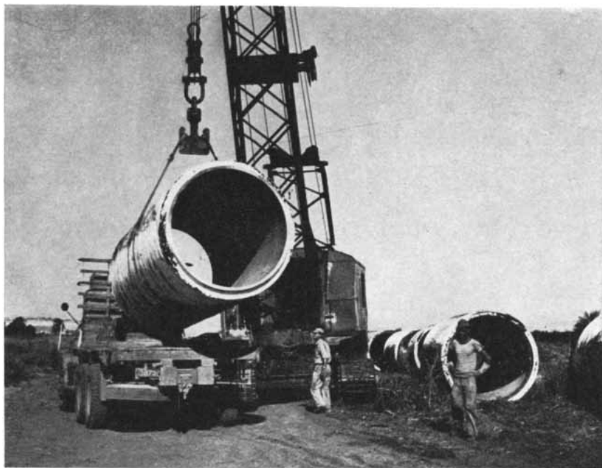
CONCRETE PIPE 70 inches in diameter for Yarkon-Negev pipeline is delivered to location where it is to be set in place in a great trench and buried. This line will carry water from the Yarkon River in the north to the arid lands of the Negev (see map on opposite page).
